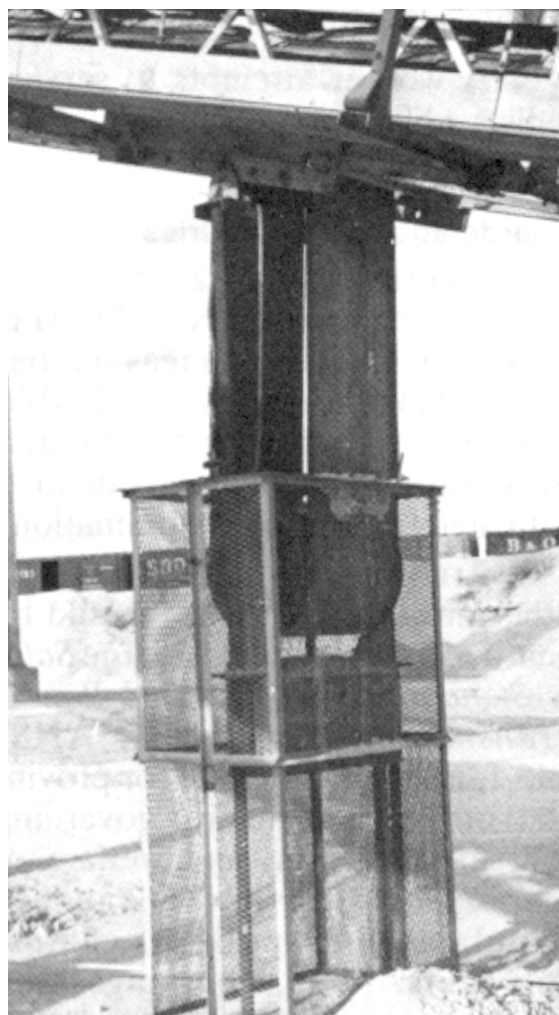
Figure 1. The belt conveyor delivers bulk material to storage piles. The belt, idlers, drive and walkway are supported by the conveyor frame.
