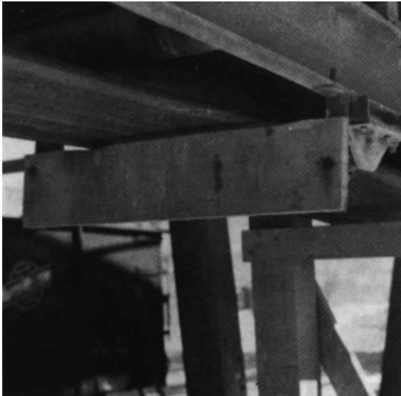
Figure 4. A simple fixed scraper will prevent build-up of materials on the belt and will do away with unsafe cleaning while the belt is moving.
